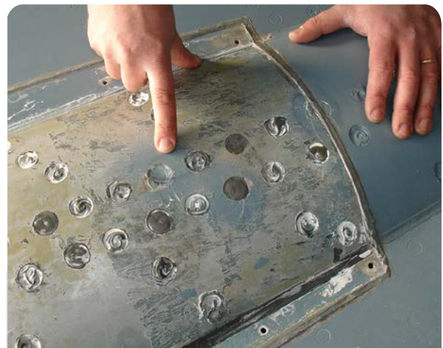
Pinpointing the leak exit point is done visually by simply observing fuel spots or drops.
