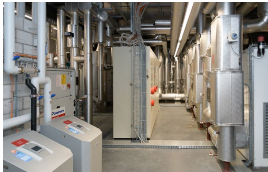
Views of the new HVAC facility, Balzers (LI)
