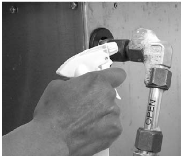
Bubbles forming at a leak.
