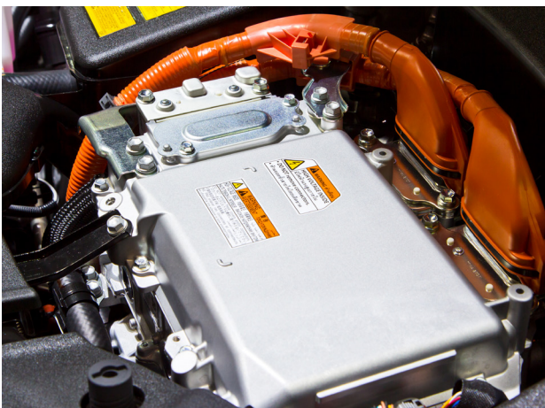
Lithium-ion batteries in hybrid vehicles.
